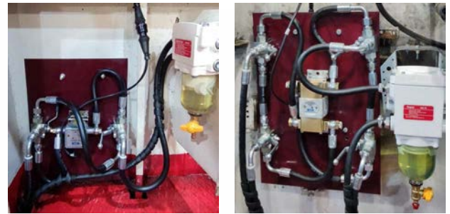
DFM 100 (on the left) and DFM 500D (on the right) fuel flow meters, installed on separate panels
