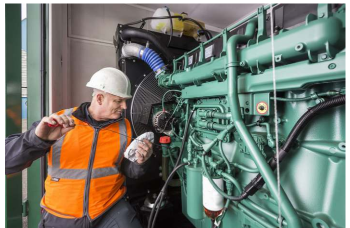
Mechanic checking the generator's technical condition
