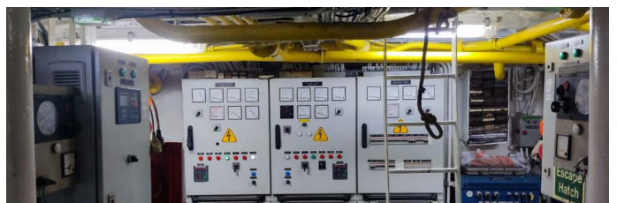
Generators and power management control panel
