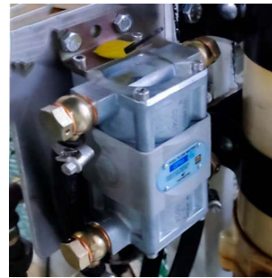
Installed DFM 250D S7 fuel flow meter
