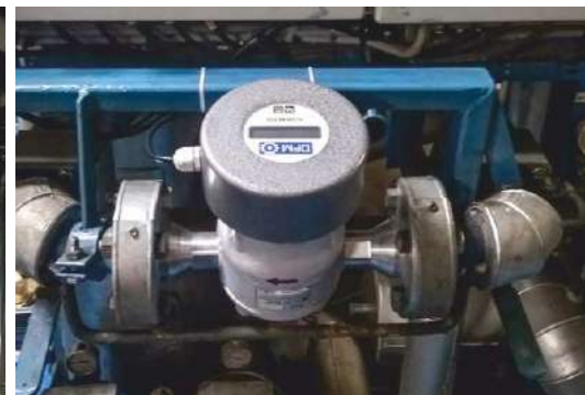
DFM Industrial flow meter, sea ferry
